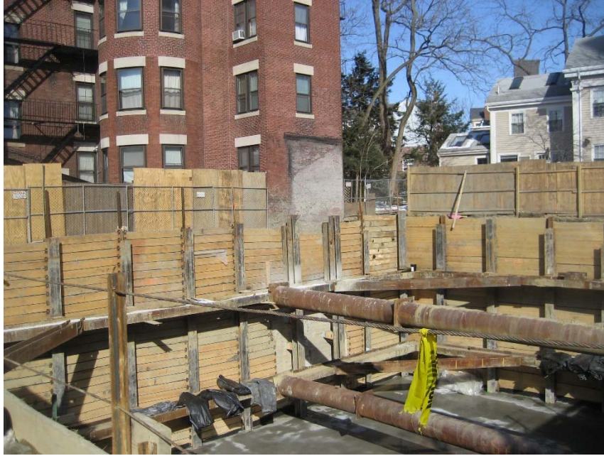
Fig. 2 – Proximity of excavation to existing adjacent structure.
